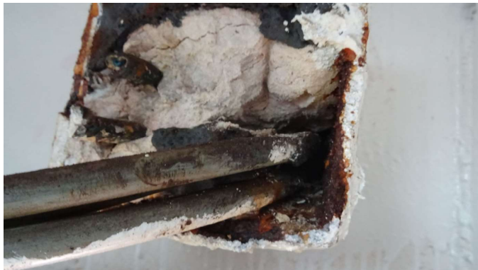
Picture 3 – self-made cable penetrations
