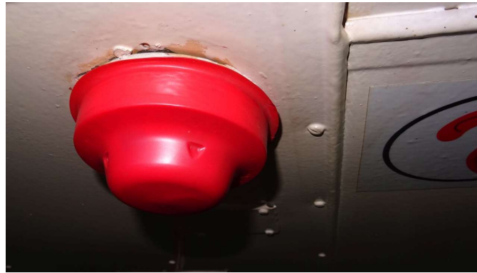
Picture 43 – disabled smoke detector in ECR
