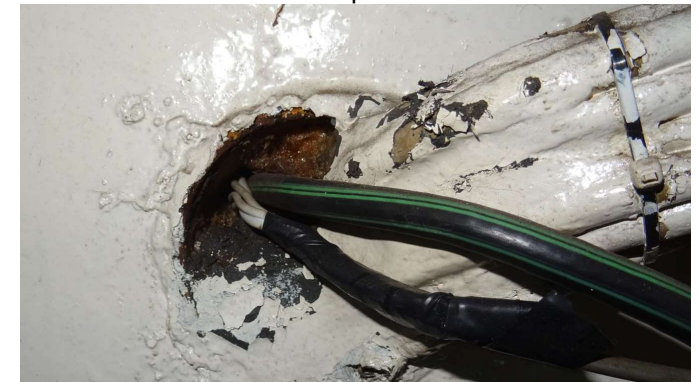
Picture 5 – self-made cable penetrations
