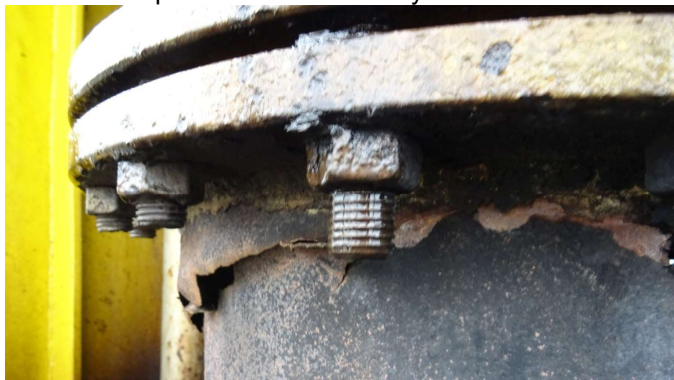
Picture 15 – the exhaust pipe found rusted through...
