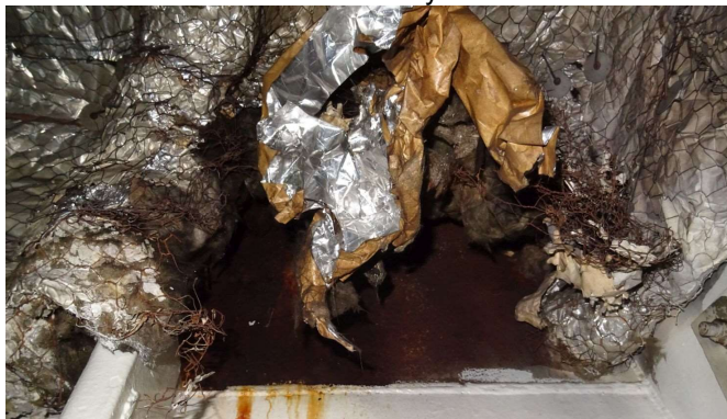
Picture 10 – ...found damaged in various spaces
