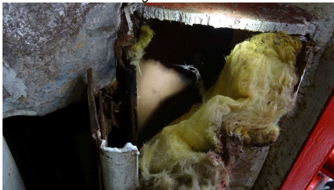
Picture 9 – The fire insulation of A60 boundaries...
