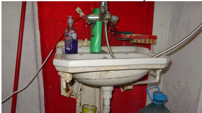
Picture 39 – self made repair by building foam and wires
