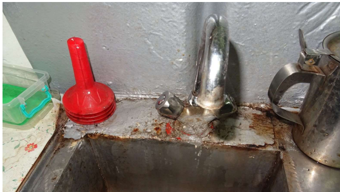
Picture 30 – self repaired washbasin
