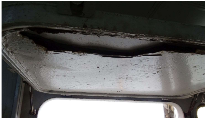
Picture 27 – ...obviously done a long time ago
