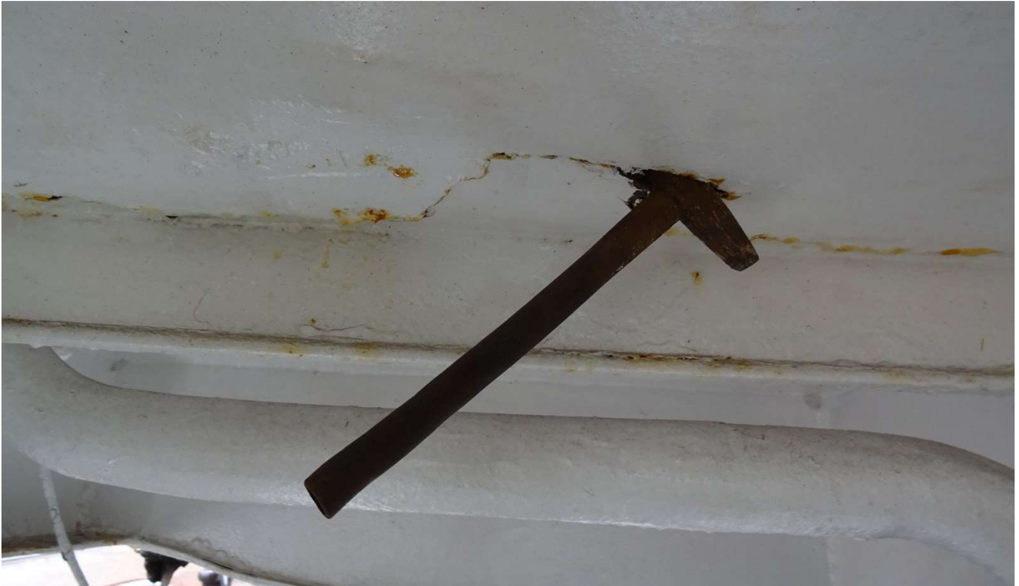
Picture 29 – testing integrity of the steel by chipping – as result severe corrosion damages were identified
