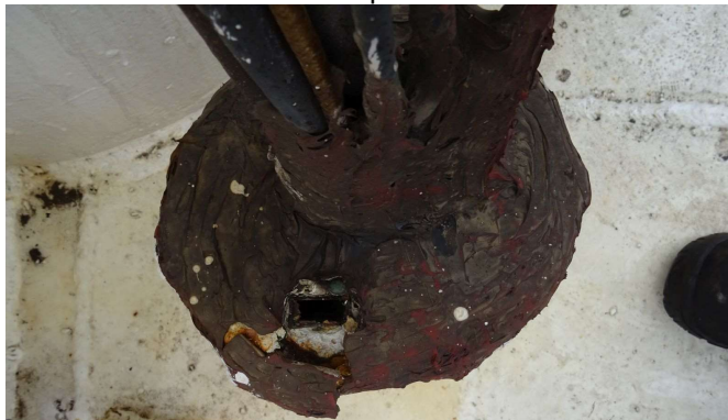
Picture 4 – self-made cable penetrations
