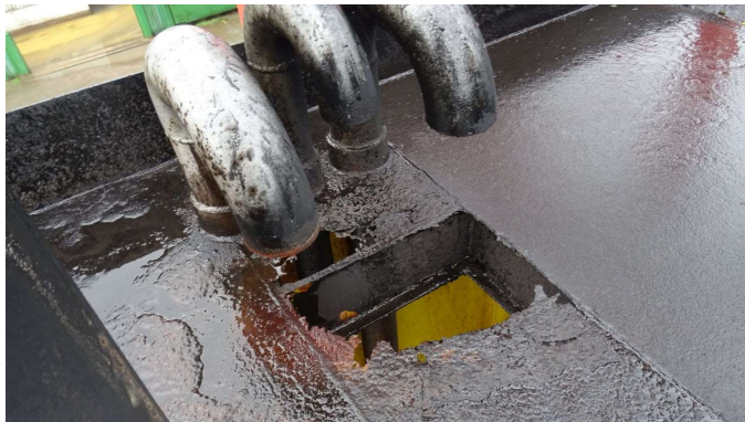
Picture 12 – platform deck holed by rust
