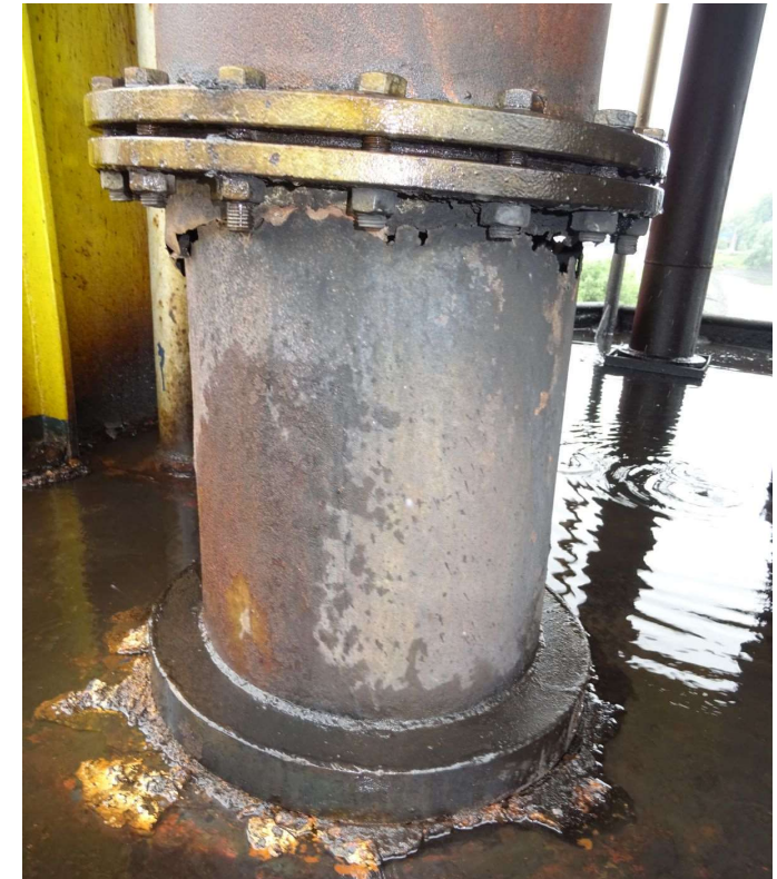
Picture 14 – rusted foundation of exhaust pipe
