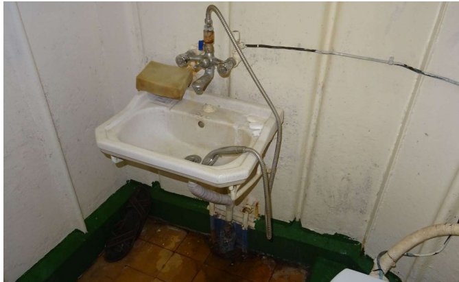
Picture 36 – The condition of the sanitary...
