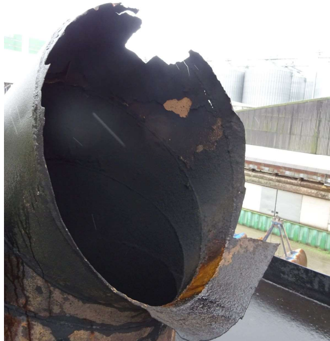
Picture 13 – funnel end rusted away
