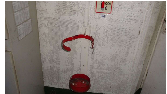
Picture 44 – missing fire extinguisher in ECR
