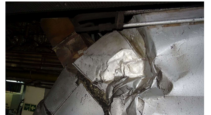
Picture 11 – damaged insulation on exhaust pipe
