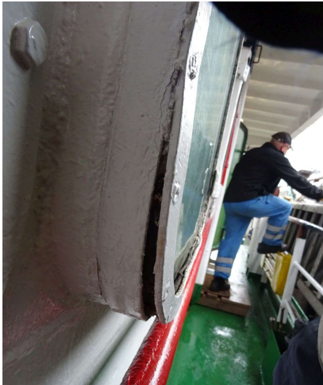
Picture 24 – window frame rusted and buckled
