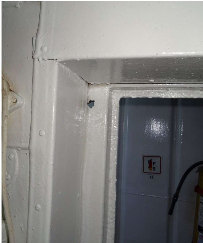
Picture 7 fire door frame holed by rust
