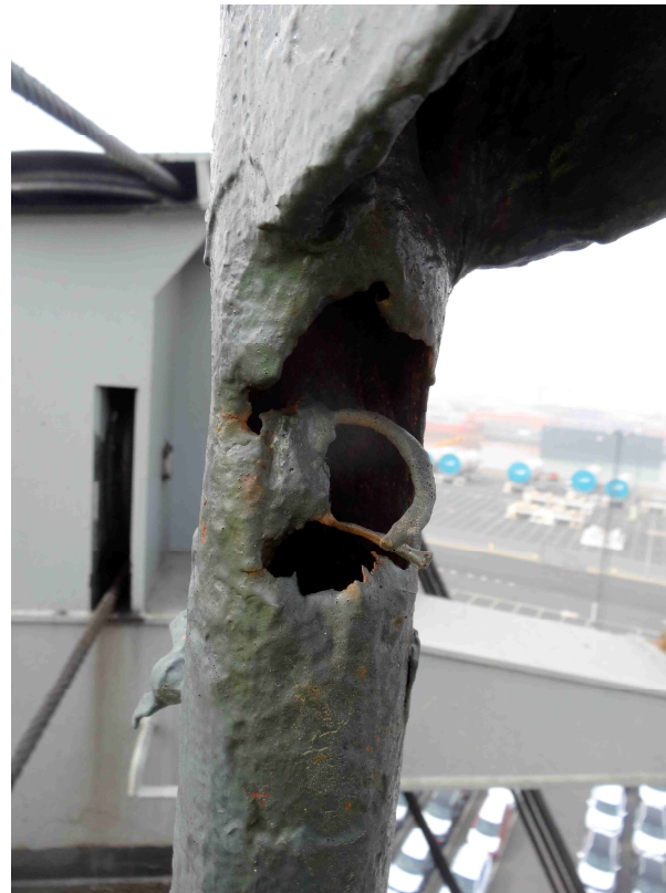
picture 2: foundation of floodlight found holed by rust
