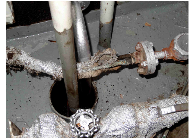
picture 20: damaged heat insulation on pipes
