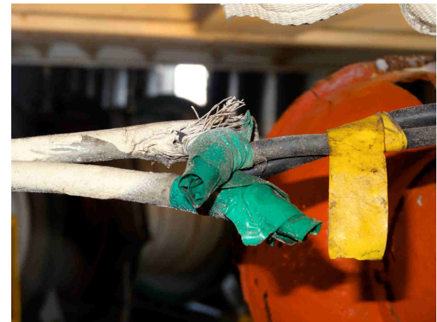
picture 17: self made professional electric installations
