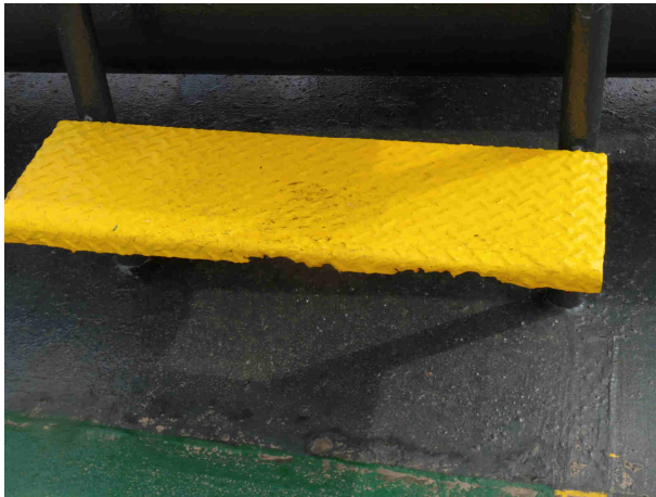
picture 12: steps and platforms were eroded...
