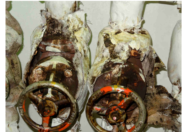
picture 21: combined: damaged and wetted through oil
