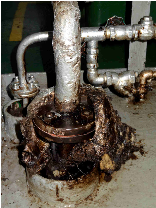
picture 22: again a combination of damaged insulation and insulation wetted through oil
