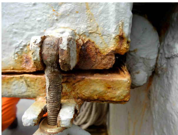
picture 1: rusted and holed fire flap
