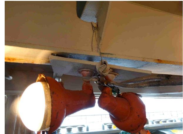
picture 16: historically grown electrical installations
